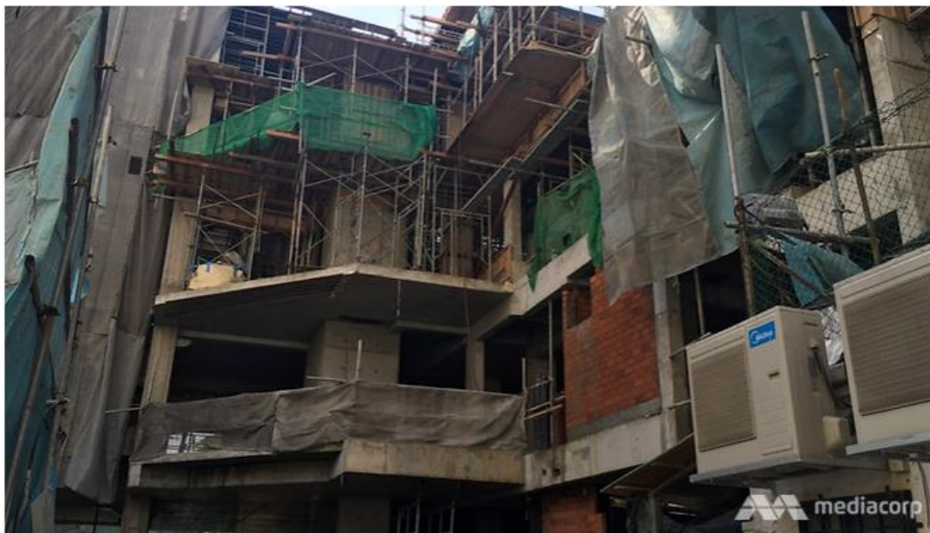
File photo of a construction site along Geylang Road without proper scaffolding and safety barricades in place. The construction company was issued a Stop-Work Order (SWO) of three weeks under new conditions imposed on May 12, 2016. (Photo: Loh Chuan Junn)
